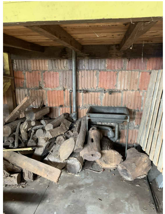
PHOTO #12 PLUMBING LOCATED WITHIN GARAGE
