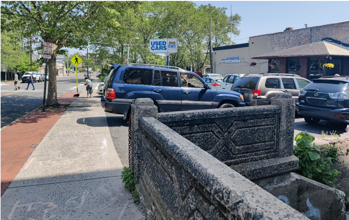
Figure 7: Car storage and open culvert along Glenridge Avenue, looking east.
