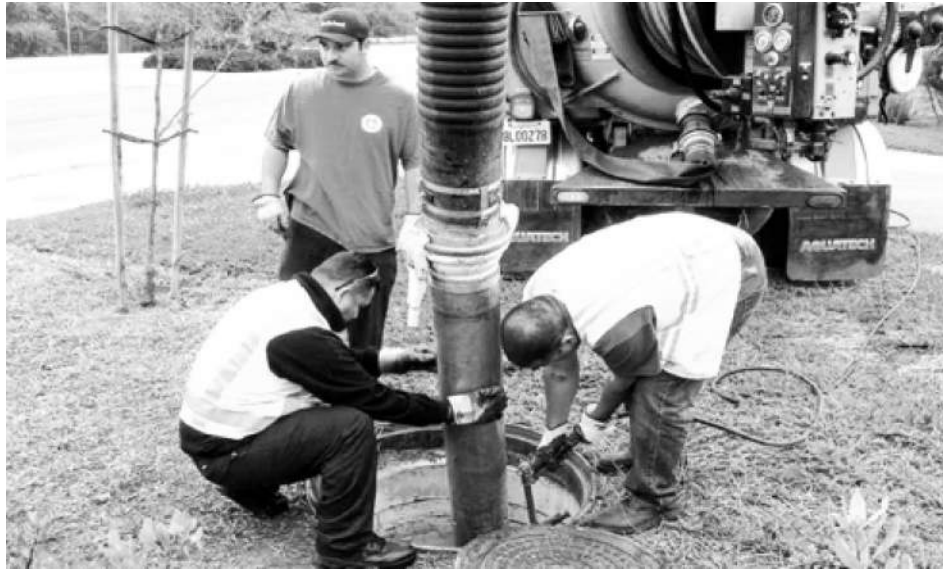
1. Remove access hatches set up vacuum truck to clean the pretreatment chamber.
